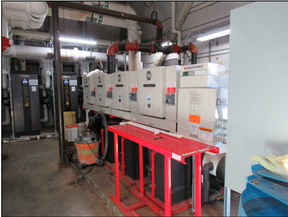
13. 200-ton Multistack chiller. Chiller was replaced in spring 2025 as part of the geothermal conversion.
