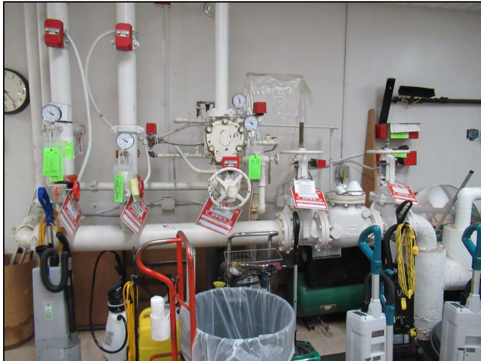
20. Fire sprinkler service risers.
