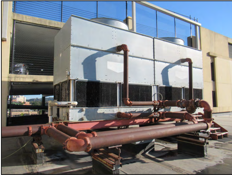
11. Cooling towers. Cooling towers are planned for removal in October 2025.
