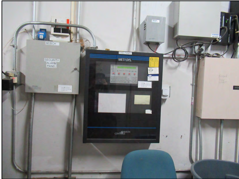
19. Fire alarm panel.
