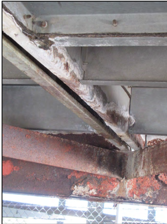
12. Rust and corrosion on the underside of the cooling towers.
