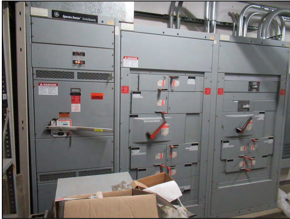
17. Main electrical service.
