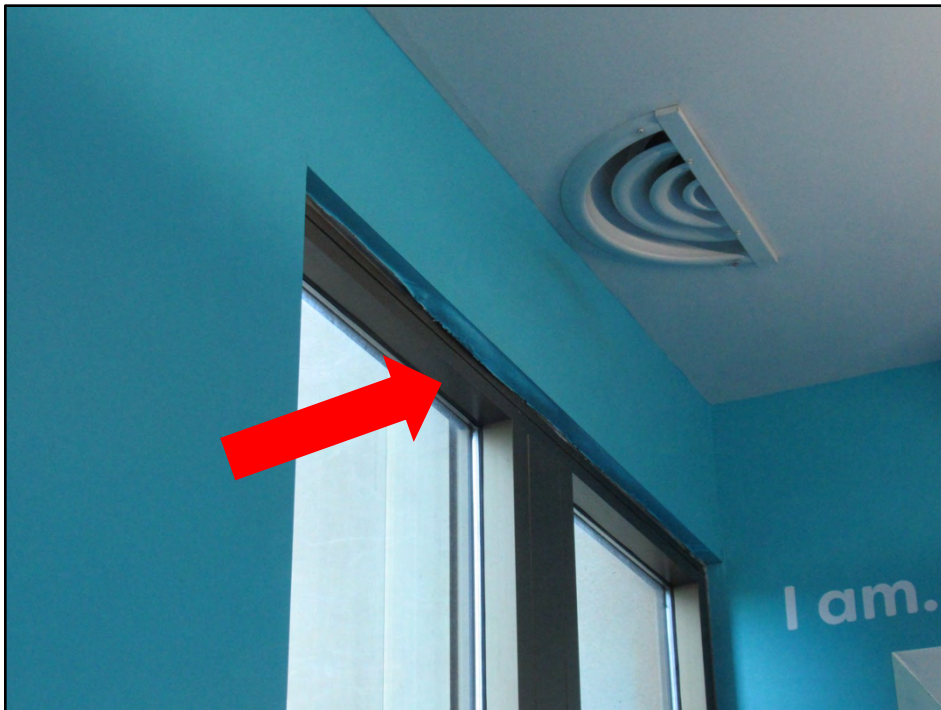
40. Water damage at Skyway.
