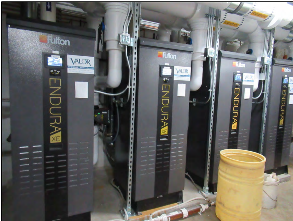
14. New natural gas fired space heating boilers.
