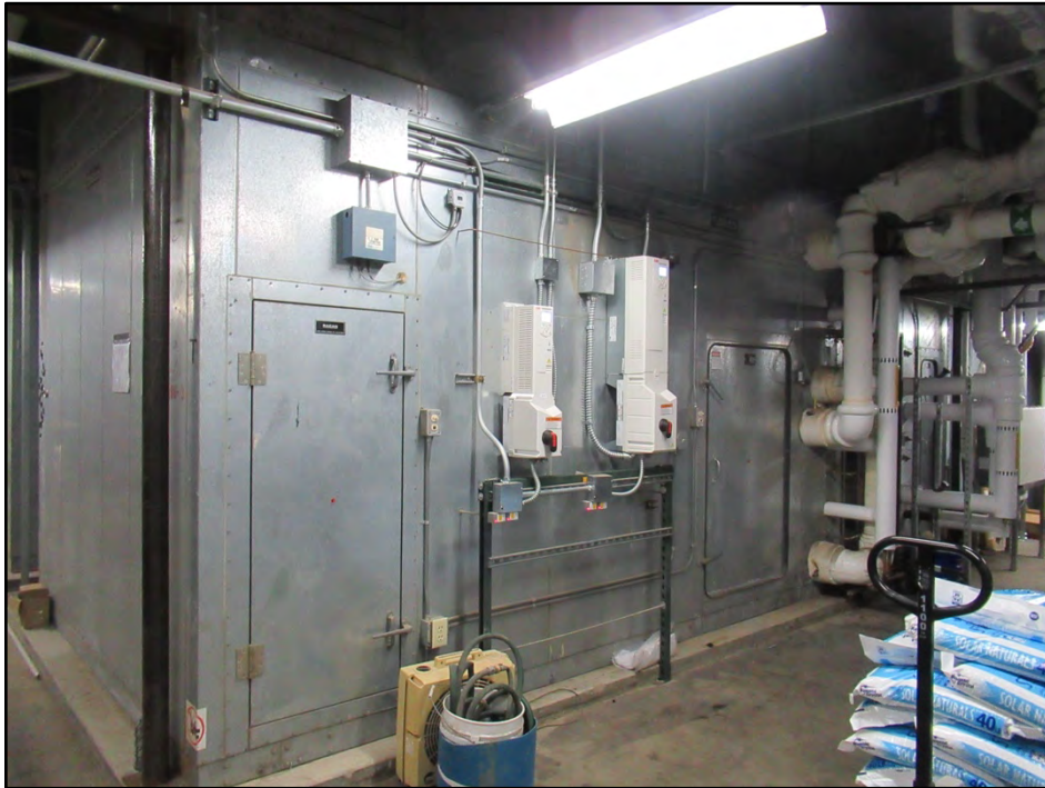
15. Typical air-handler, one of four.
