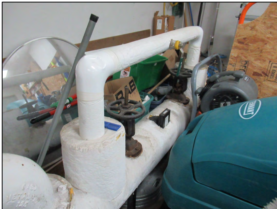
21. Domestic water service.
