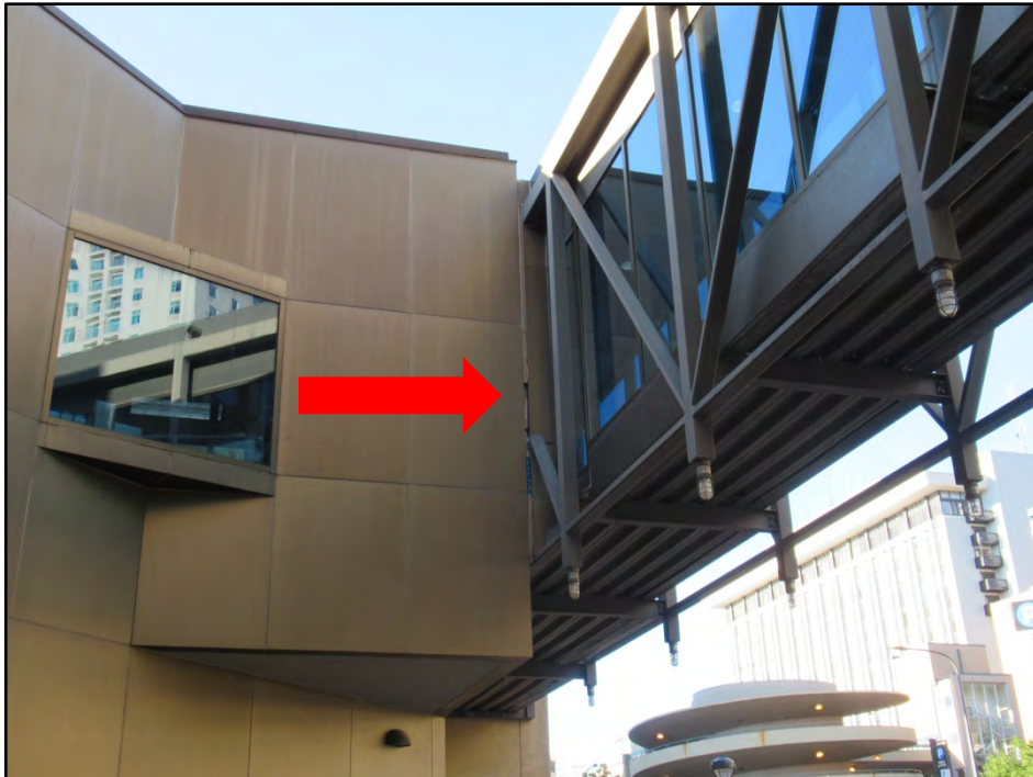
38. Library and Skyway intersection with missing flashing.
