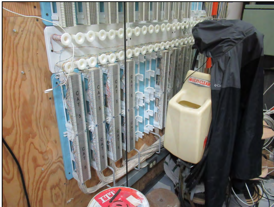
22. Telephone service MPOE.
