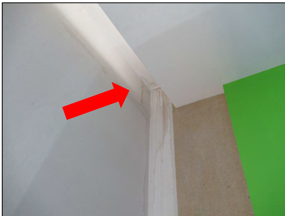
41. Water damage at the Skyway.
