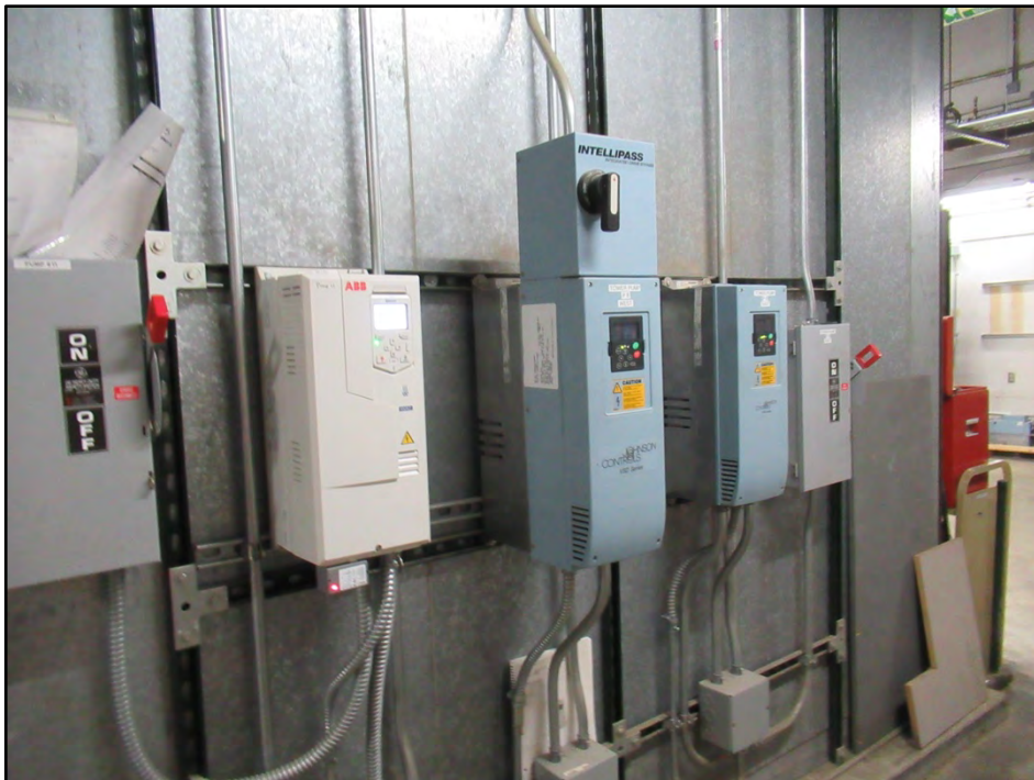
16. Typical variable frequency drives.
